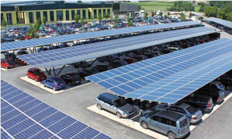
↑ solar generation within car park areas
